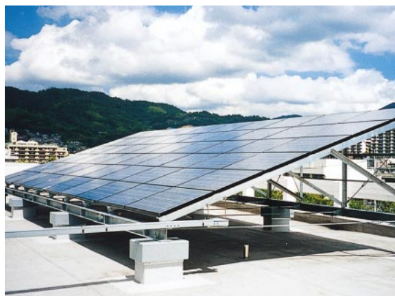
Solar Power Generation System (Kure Technical College)
