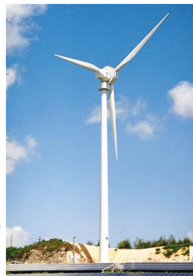
500kW Wind Power Generation System (Okinawa Electric Power Company)
