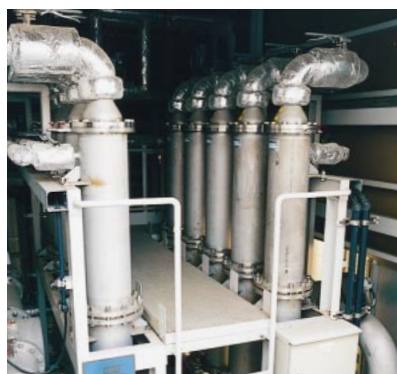
Using a membrane filter, this wastewater treatment device at Hitachi's Naka semiconductor production facility plays a crucial role in the recycling of wastewater.
