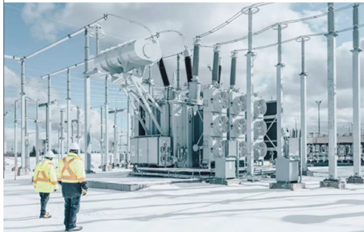
Efforts aimed at transformer recycling
